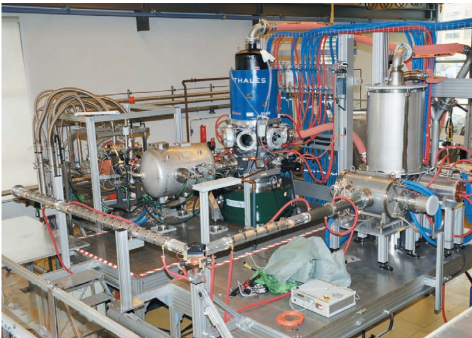
The two gyrotron towers of the test facility at SPC. Both gyrotrons are ITER-class, 1MW, 1000s, 170GHz tubes, similar to those that will power one of the 8 beams of the ITER Upper Launcher, seen on the opposite page. The left one is the EU gyrotron manufactured by THALES, the right one is the gyrotron manufactured by GYCOM used to test components of the ITER Upper Launcher.
